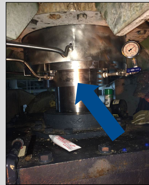
After: Pulper drive shaft with Inpro/Seal Air Mizer shaft seal in operation
