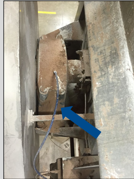
Before: Leaking Contact Seal
