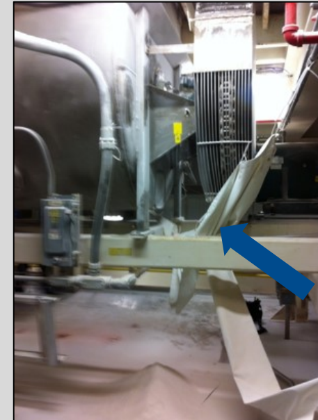
Before: Tarp installed to help catch leaking pancake mix
